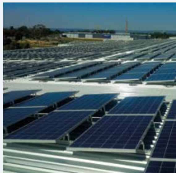
Solar installations on all new group builds.
